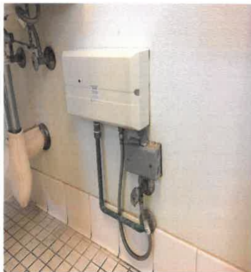
Water Heater for Restroom Lavatory
