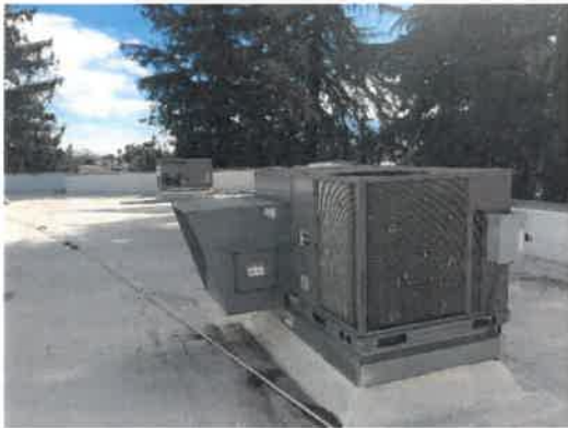
Typical RTU unit
