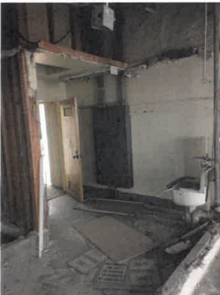
Existing Panelboard in Janitors Closet
