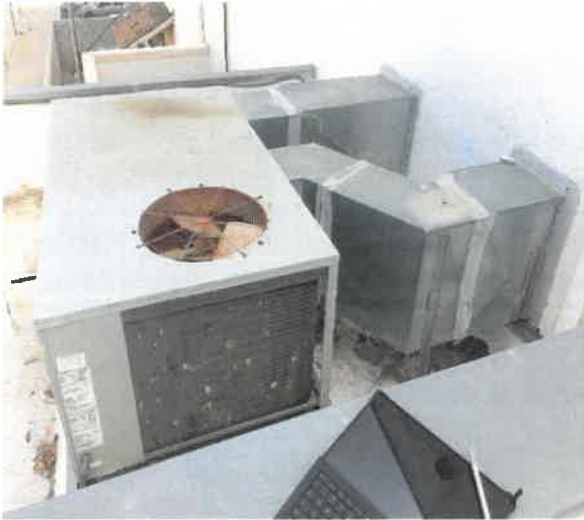
Roof Mounted Unit Serving Gym
