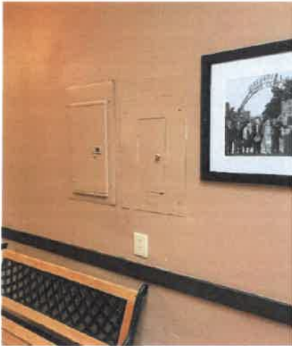
Existing Panel being used as junction box
