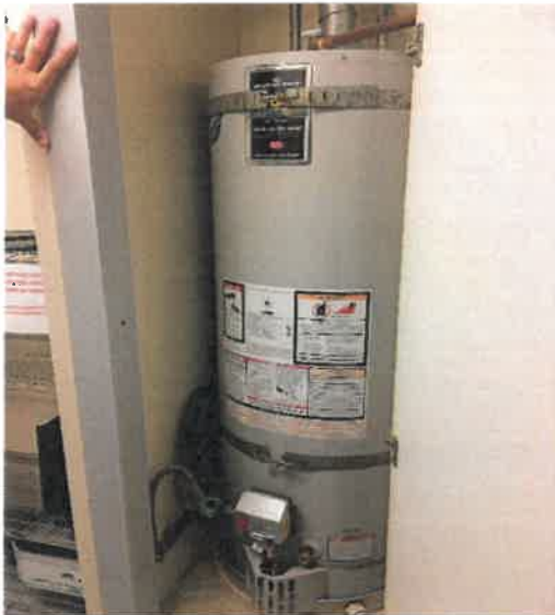
Water Heater for Kitchen
