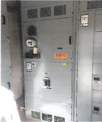
Existing Main Switchgear
